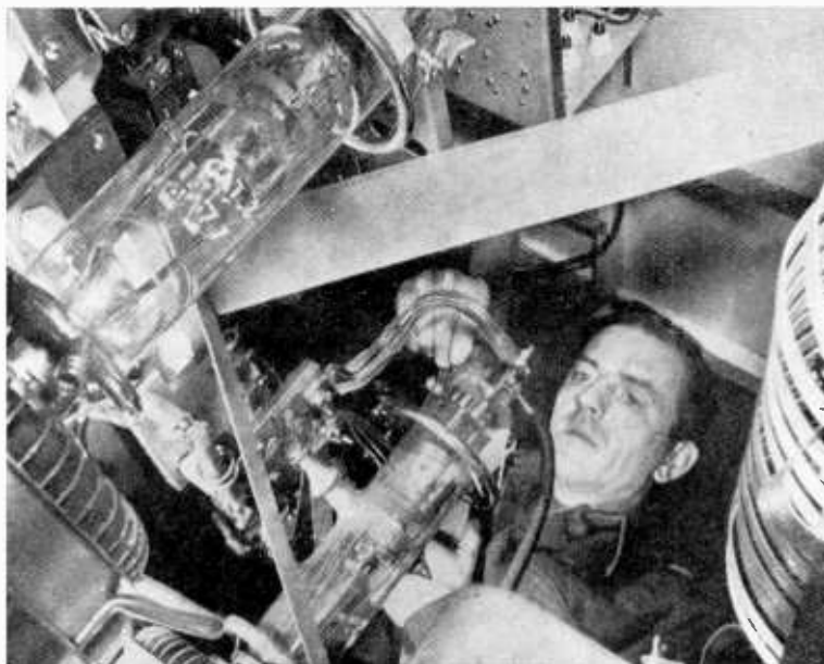
Royal Canadian Air Force photograph The filament leads being replaced on an air-cooled CAT3 valve on arrival at a new site
